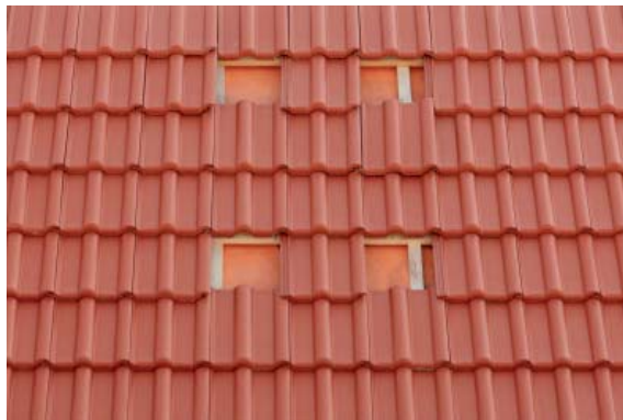
Figure 2: Pushed up roof tiles
